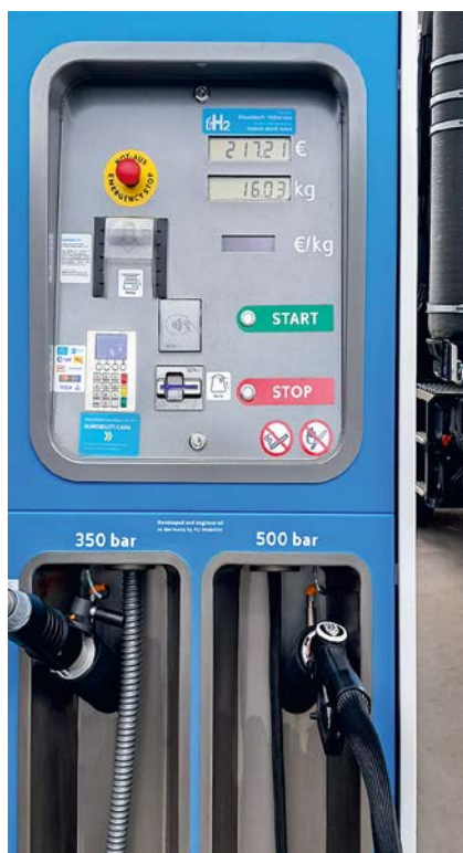
At one of the three dispensers in Düsseldorf, 500-bar hydrogen can also be refueled.
