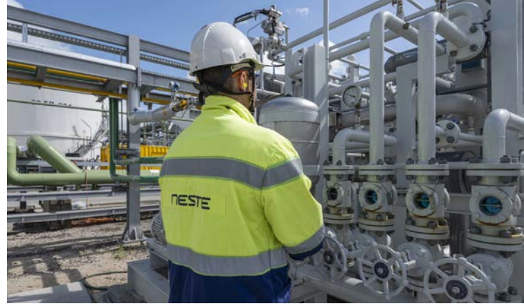
The high-temperature electrolysis system has been integrated into the processes of the Neste refinery in Rotterdam. © Sunfire
